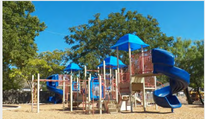
Renovations to the playscape at Little Zilker Park included a full equipment change-out.
