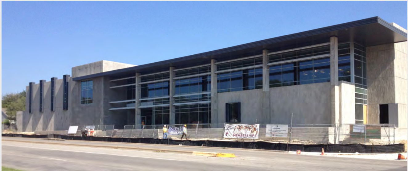
The new North Austin Community Recreation Center was built in partnership with the YMCA, and funded in part by funds from the 2006 Bond Program.
