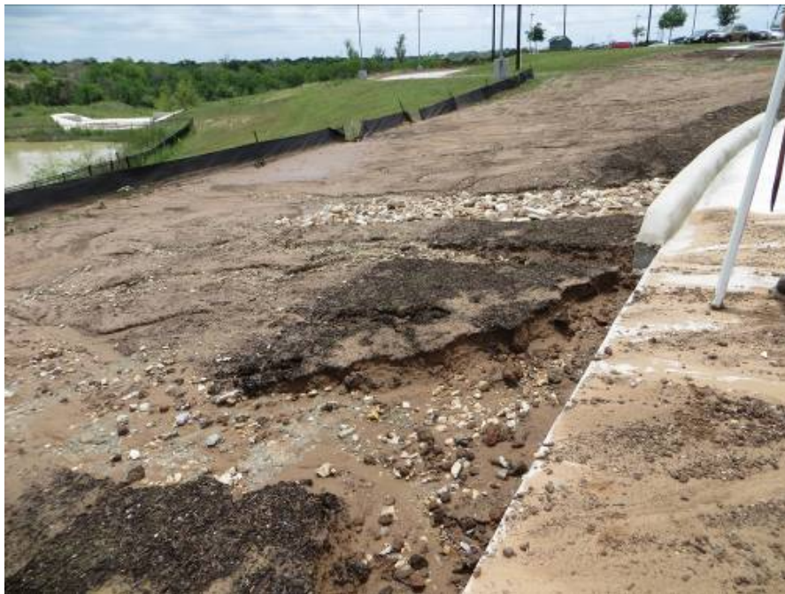
Active Surface Erosion from Unvegetated Areas the Recreation Center
