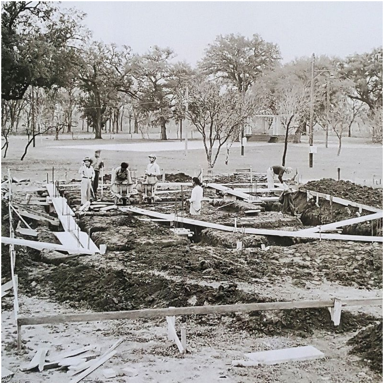
Figure 19. Swimming pool construction, ca. 1933. Jen Massing-Harris, "Parque Zaragoza Neighborhood Park Pool & Bathhouse Caretaker Cottage Updates," September 24, 2019, http://www.zarozaparkneighborhoodassn.org/neighborhood-nose-sniffing-out-the-scoops-for-the-east-austin-parque-zaragoza-community
