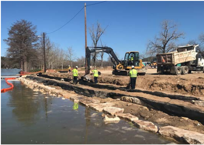
Figure 8. The progressive vision for the shoreline materialized as crews from the Field Operations Division demolished the old wall and installed the new structure during the winter of 2017.
