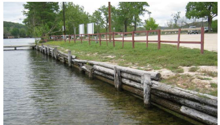
Figure 6. The decaying wall at Emma Long Park had degraded the shoreline and was not compliant with current City code.
