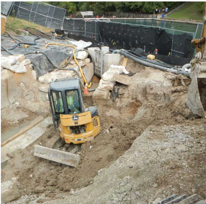
Figure 12. Eliza stream construction showing wall foundations, rock walls for the slope and stream channel, and stream channel being built
