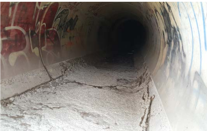
Figure 6. Milk sludge trapped in storm pipe
